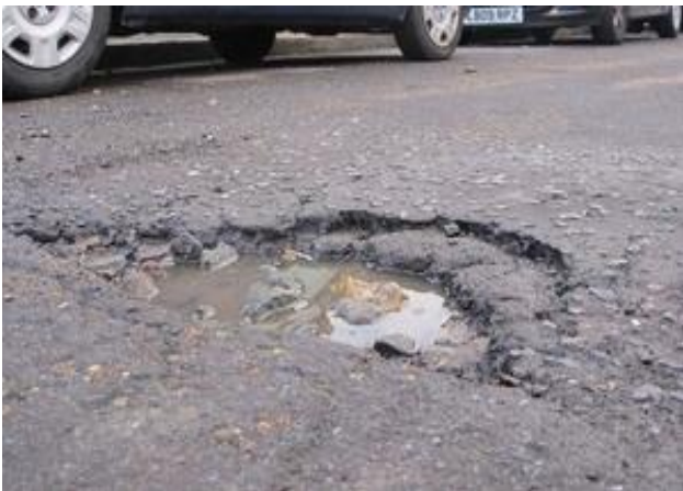
Figure 4. Pothole on a road
