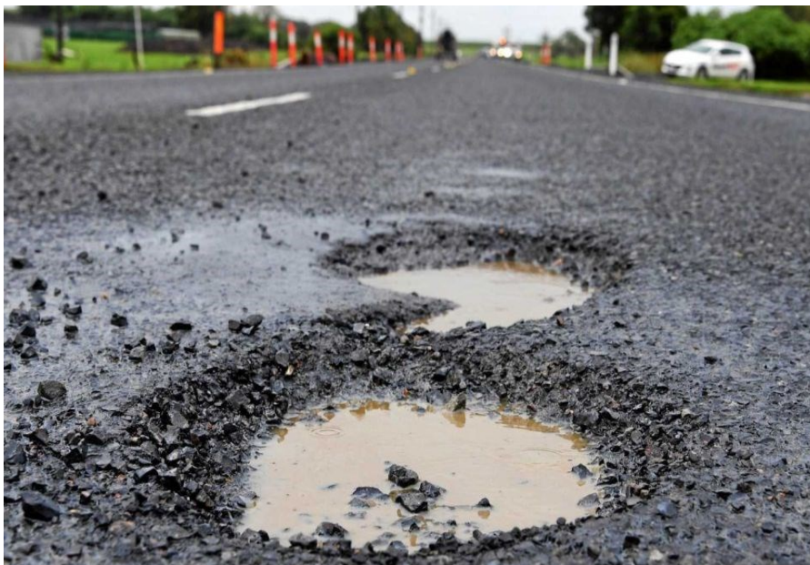
Figure 1. Road problems damage vehicles and cause traffic accidents.
